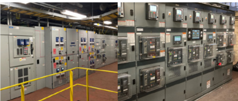
Figure 20. No. 1 Control Room and 25-Cycle Switch Gear Projects.
