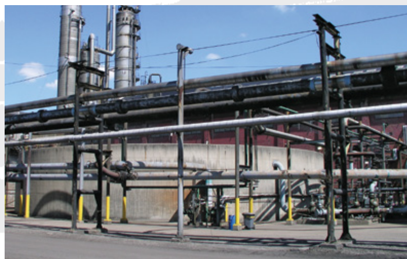
Figure 28. Biological Plant Ammonia Stills and Clarifier.
